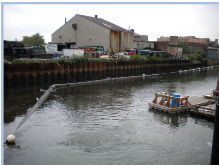
Exposed Diffuser Pipe at Low Tide
