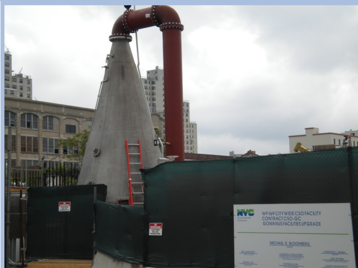
Installation of ECO 2 's Speece Cone at Gowanus Canal
