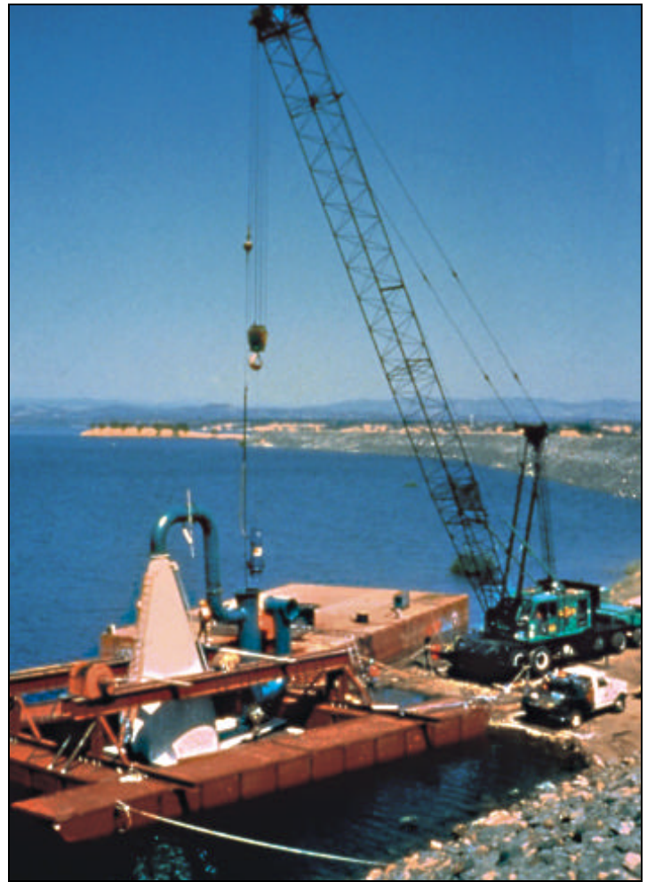
A Flygt propeller pump combines oxygen and water in this 23-foot tall, cone-shaped oxygenator.
